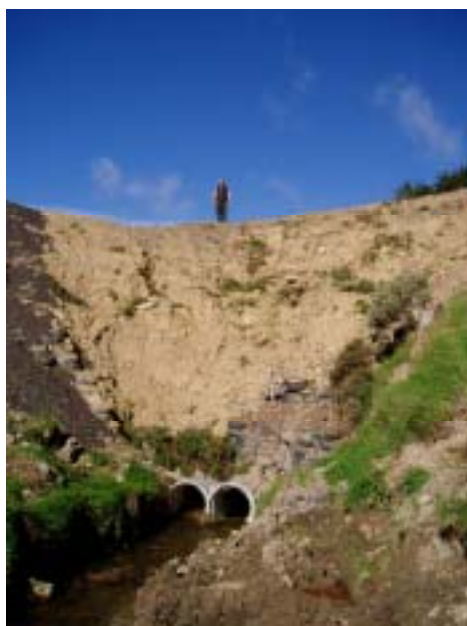
Unconsented culvert and crossing installed on the Ohariu Gorge, Wellington.
