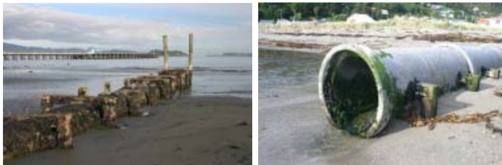
Figure 4.15: Stormwater outfalls at Petone Beach (left) and Rona Bay at the northern end of Cliff Bishop Park.
