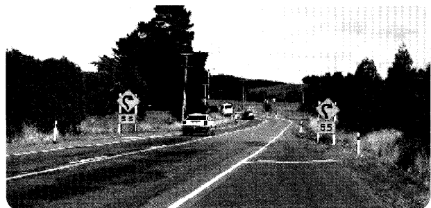
Photos left and above: Kaitoke Hill Upgrade on SH2, linking Wairarapa and Wellington
