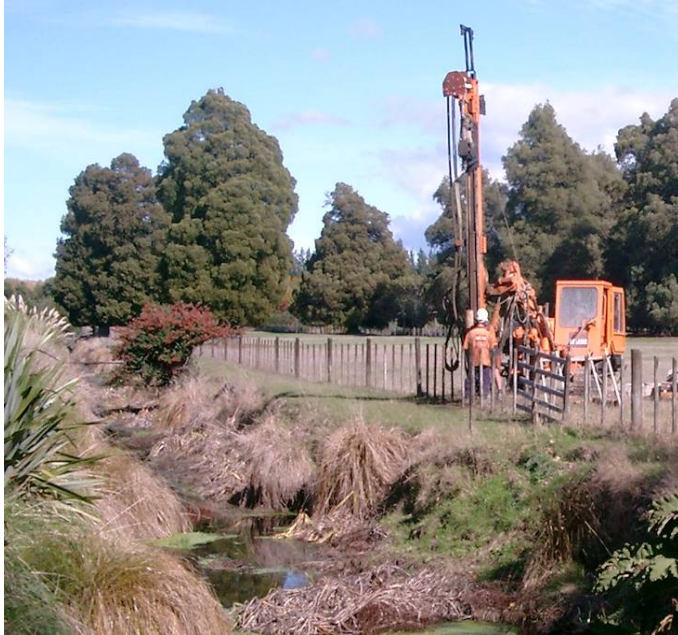
Figure 4: Example of recent field work with the drilling of a new monitoring borehole at Poterau Spring in the Te Ore Ore east of Masterton. The groundwater-fed stream in the foreground has been progressively drying up during summer months from year to year due to lowering groundwater tables. This new borehole and others installed across the valley will help improve our understanding of the complex connections between groundwater and surface water.
