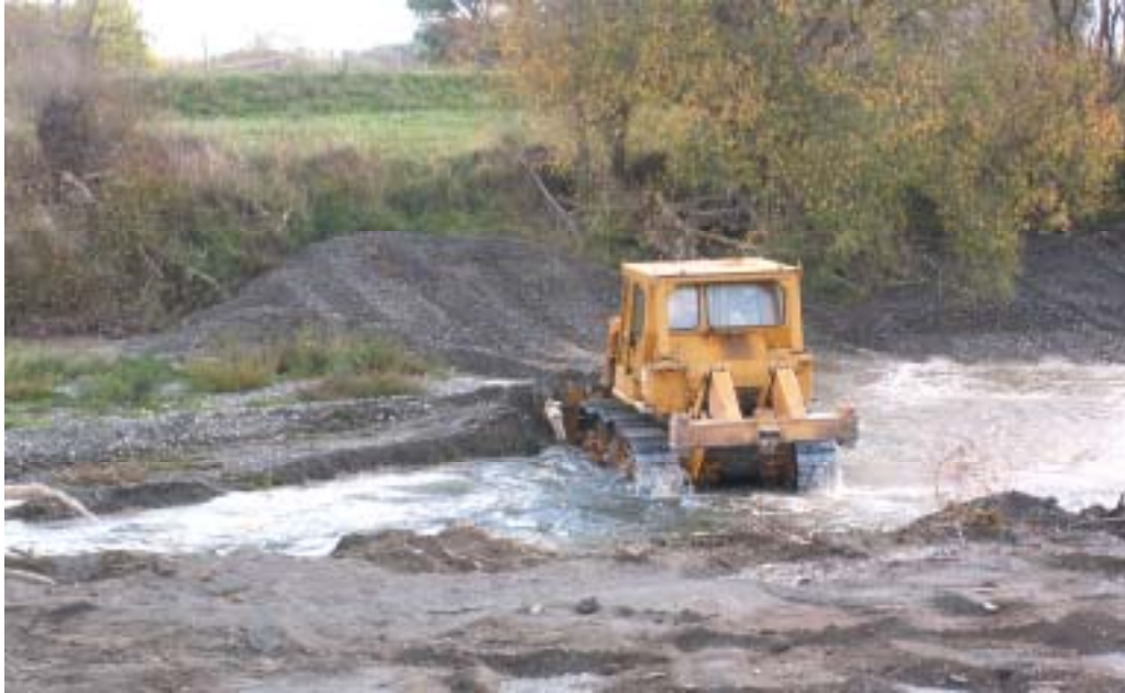
Illegal river works on Huangarua River
