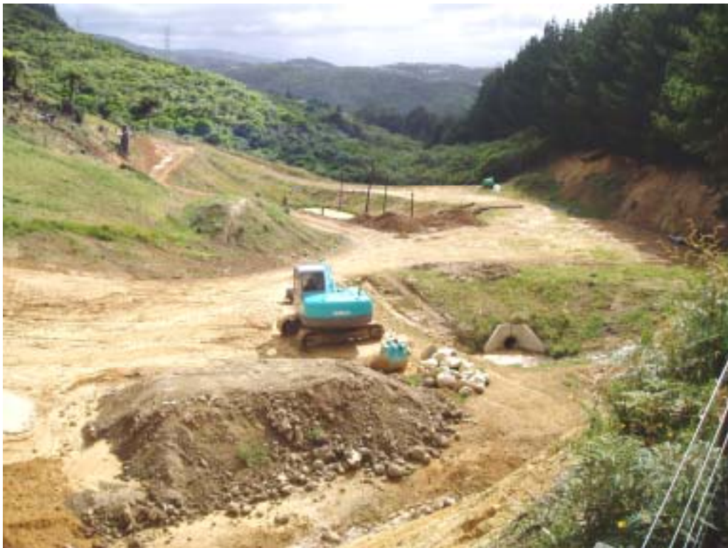
Unconsented vegetation clearance in Hutt City
