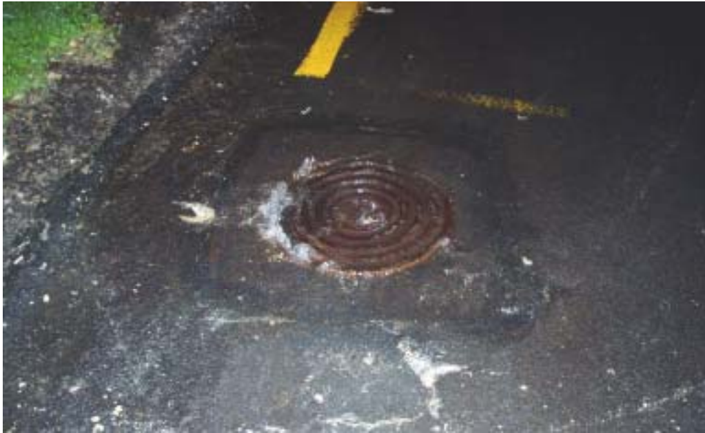
Sewage overflow in Petone
