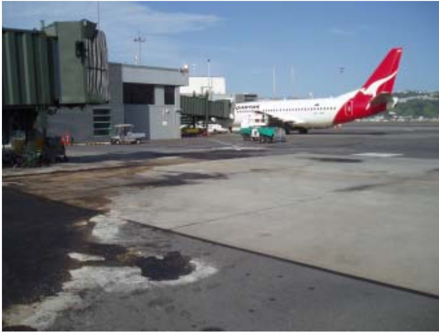
Fuel spill from Aviation Ground Services in Miramar
