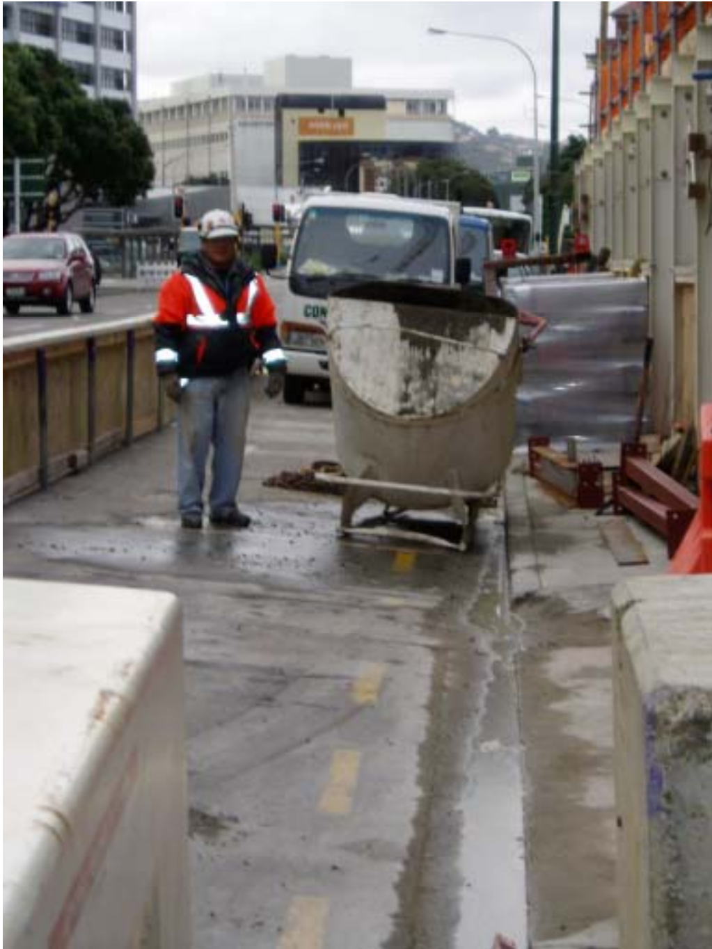
Discharge of liquid waste to stormwater in Wellington City
