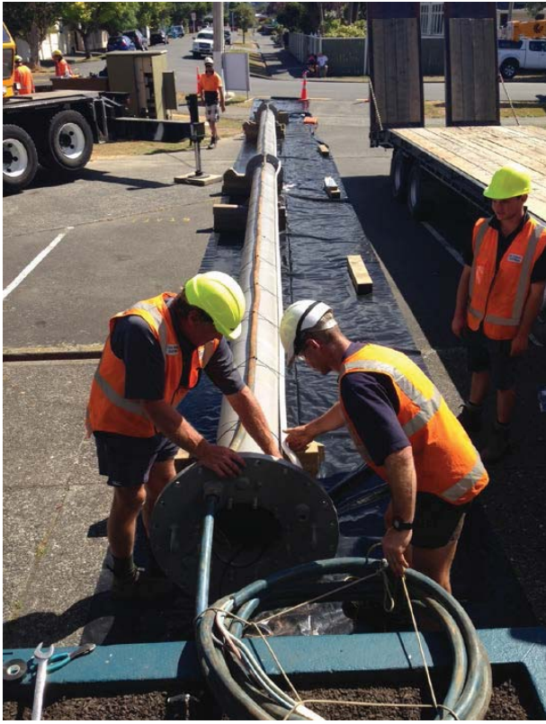
After the Waterloo well affected by iron bacteria was cleaned, the bore's pump is attached to a 16m positioning pipe in order to be lowered back into the aquifer.
