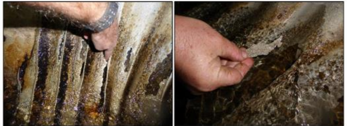
Figure 4: Localised Abrasion Damage found by Damwatch (2015)
