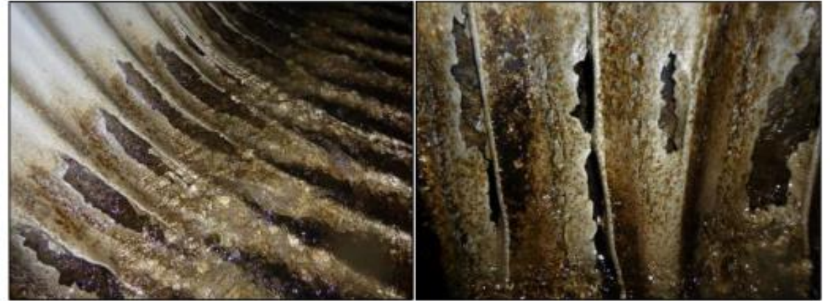
Figure 3: Localised Abrasion Damage found by Damwatch (2015)
