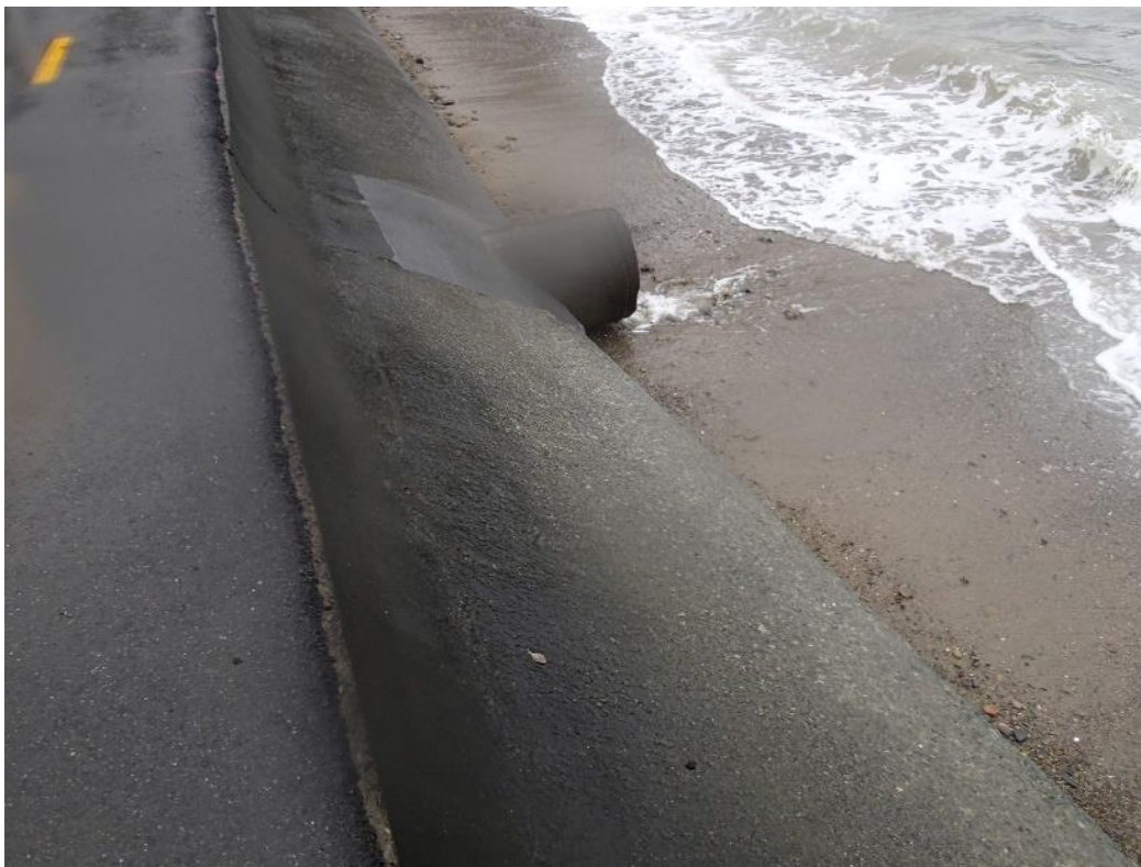
Figure 9-2: York Bay North stormwater outlet. Photo P6230205, 2017-06-23, taken 4 hours before high tide on 1.3 m tidal range.
