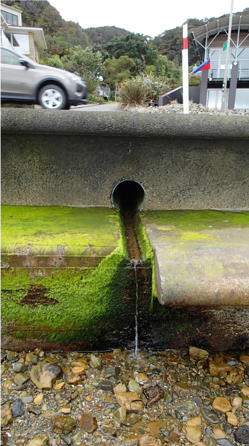
Figure 8-3: Stormwater pipe used by little penguins, Wilmore Way, northern end of Whiorau/Lowry Bay. Little penguins were reported in this drain on the inland side of the road in May 2017. The 60 cm vertical rise is a direct access barrier to the drain when the tide is low, but unimpeded access may be gained via rocks to the left (not shown). Photo: PA060034.JPG, 2016-10-06.
