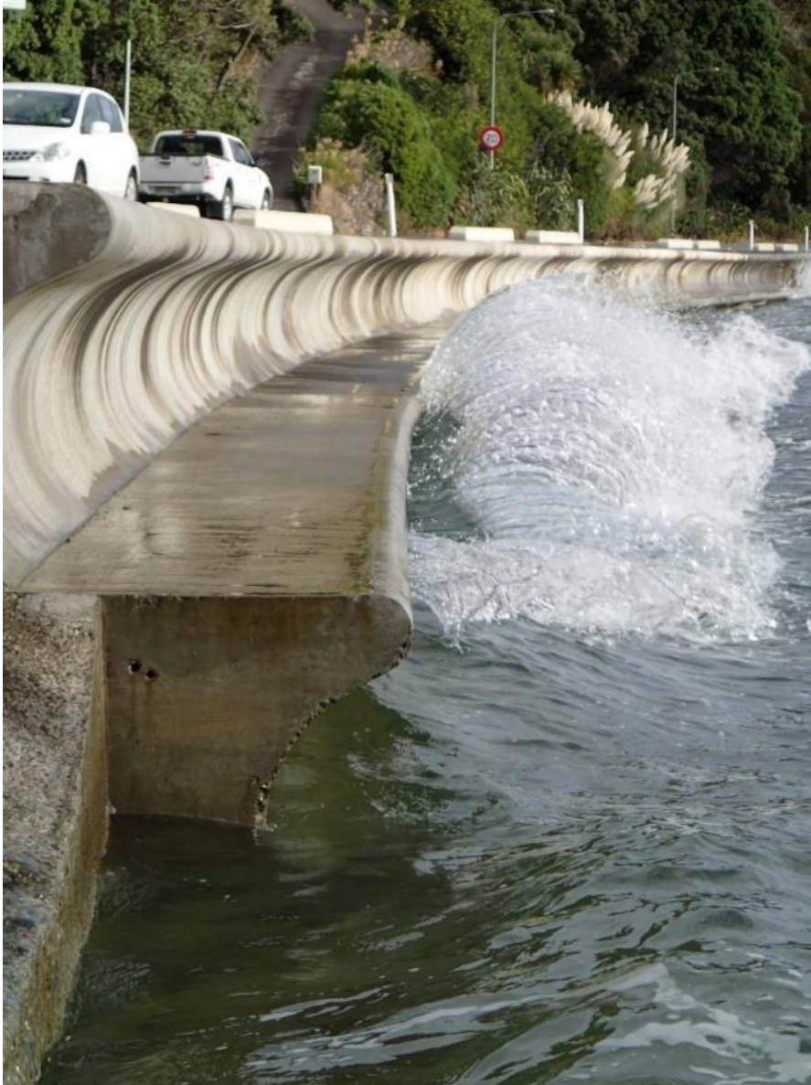
Figure 7-1: Existing double curved seawall, York Bay, built 2007–2008. Photo (taken close to high tide) illustrates loss of a narrow zone of intertidal habitat, and outcomes against hard protection structures (that will increase with sea-level rise). Textures are proposed to be incorporated into one curve face (5 mm depth) and a flat step (50-70 mm depth) to enhance habitat complexity and protection for biota. Photo: P5040292, 2016-05-04
