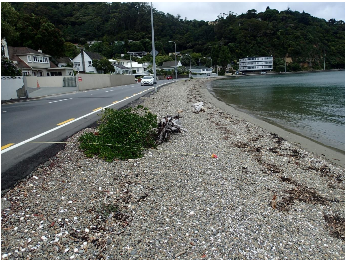
Figure 2-1: Proposed 3.5 m shared path width (indicated by tape measure), 45 m south of Cheviot Road bus stop, Whiorau Lowry Bay. The toe of the single curve seawall here would extend a further 600 mm seawards from the tape measure end. The effective encroachment distance (from toe of existing low seawall to toe of proposed new seawall) is 3.1 m. Photo: PC310808.JPG, 2018-12-31, 15 minutes after high tide.
