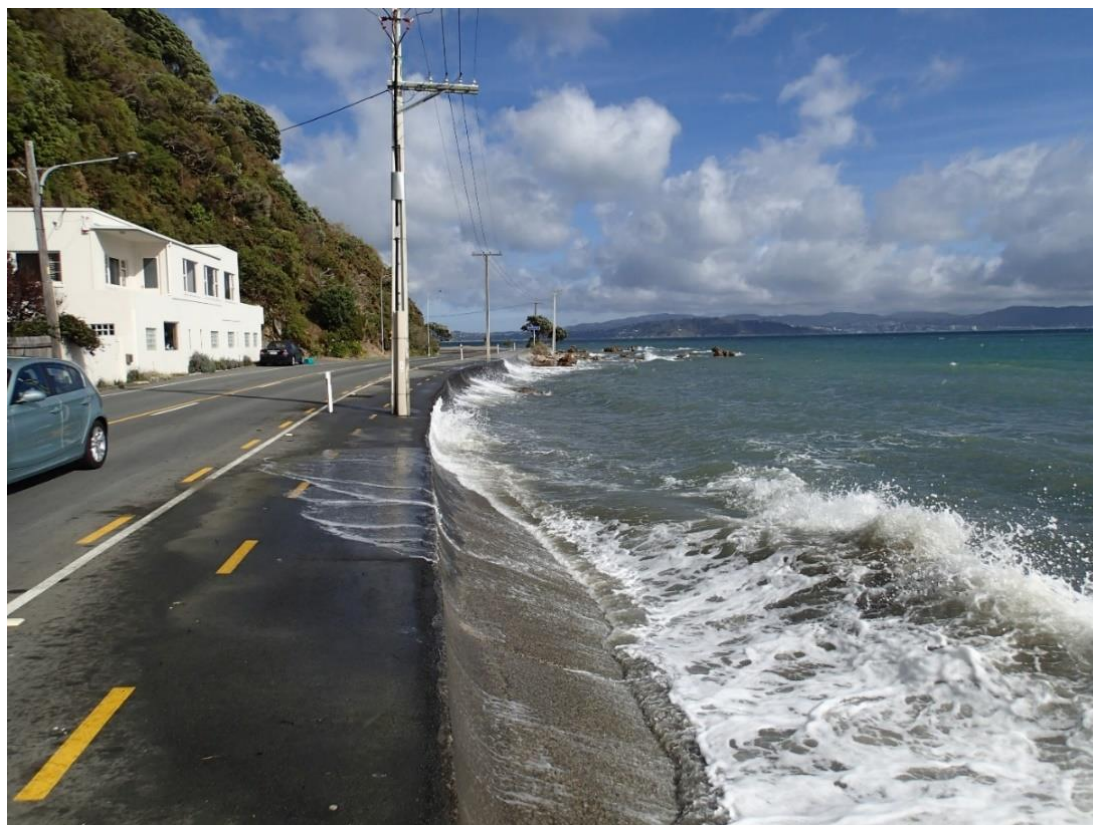
Figure 8-2: Older style angled concrete seawall, Mahina Bay. The steep riser up to the road is likely to be a difficult or impassable barrier for little penguin access. Photo: P5020130, 2016-05-02.
