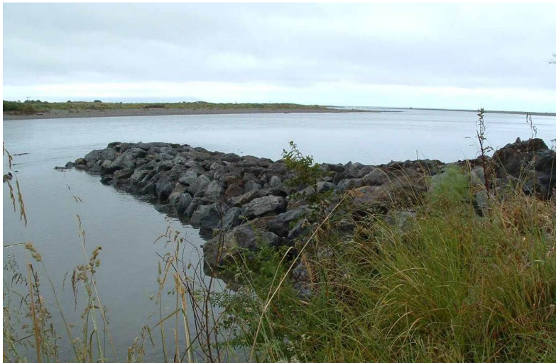
3 Completed groyne (XS 70 approx)
