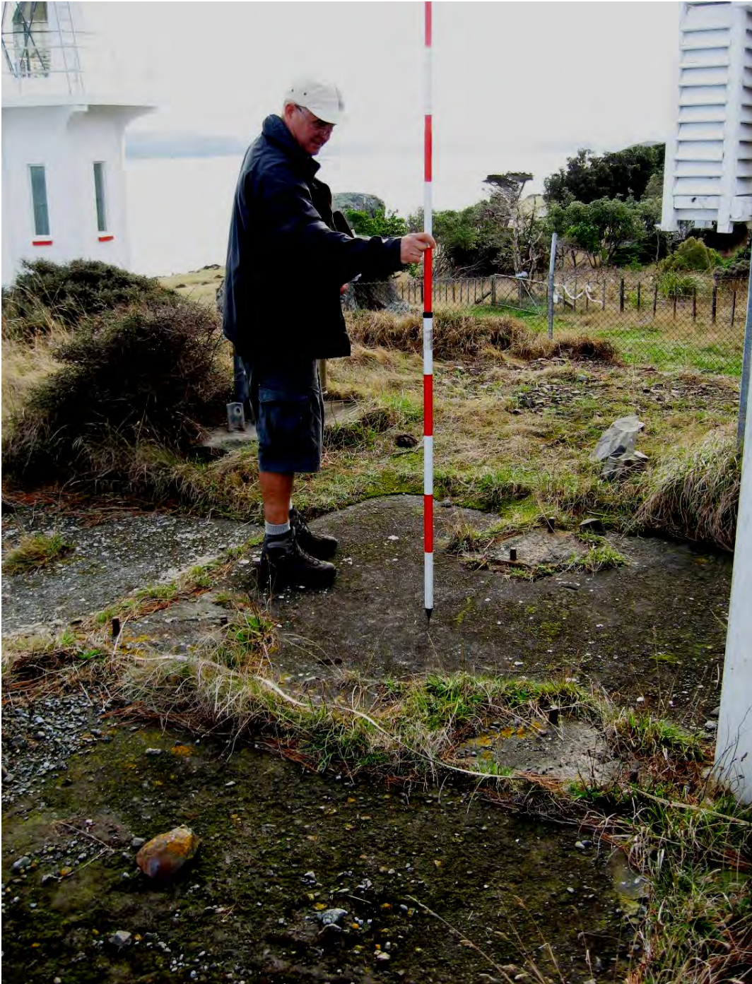
Fig. 21. The radial arrangement of bolts for the brackets holding the signal mast.
