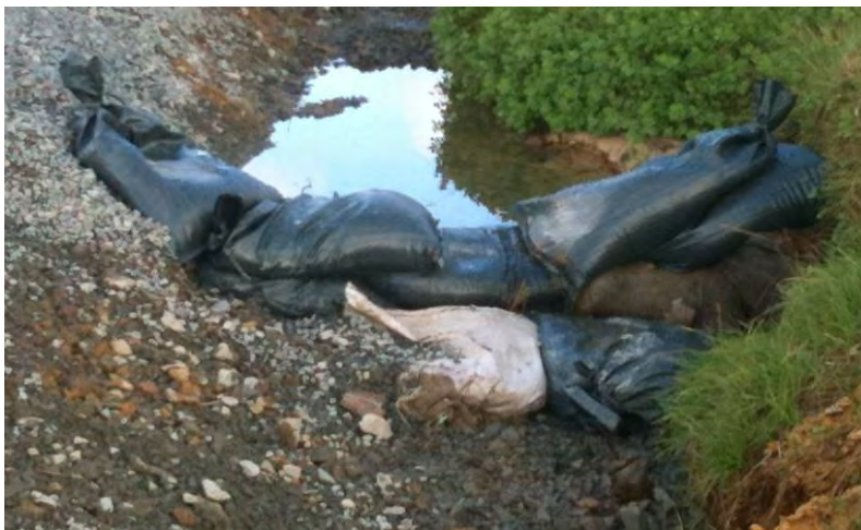
Figure 28: Check dams installed with a spillway to direct flows over the centre of the structure. Sand bags placed directly below spillway provide a protective apron below the dam
