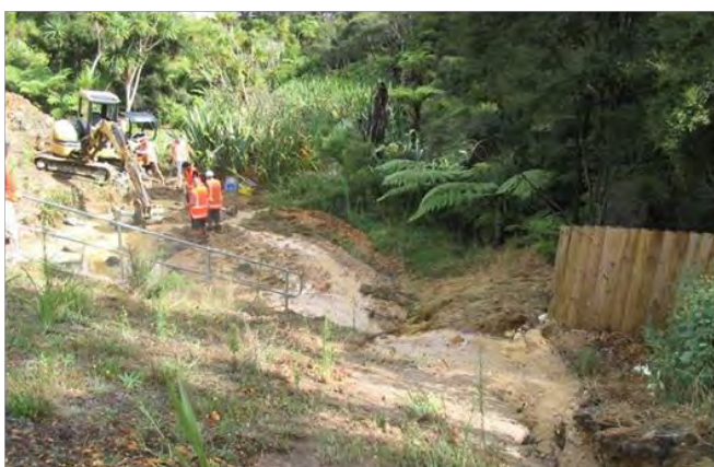
Figure 13: Sediment discharge as a result of not protecting the watercourse
