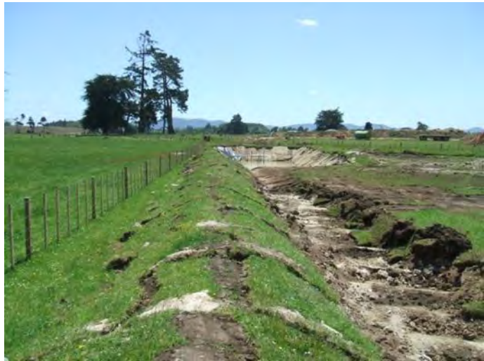
Figure 16: Turfing scraped from within the site to stabilise the perimeter bund. The perimeter bund provides both clean and dirty water control
