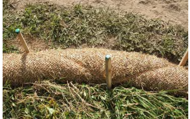
Figure 94: Straw sock secured in place using stakes and bale twine; note the stakes are placed every 600 mm
