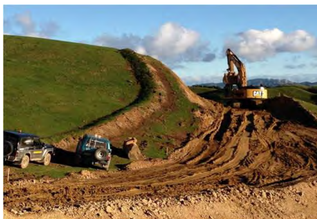
Figure 15: Clean water diversion used to isolate upper clean water flows from the works area
