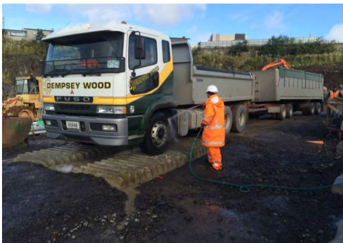
Figure 37: Example of truck wash and shaker ramp
