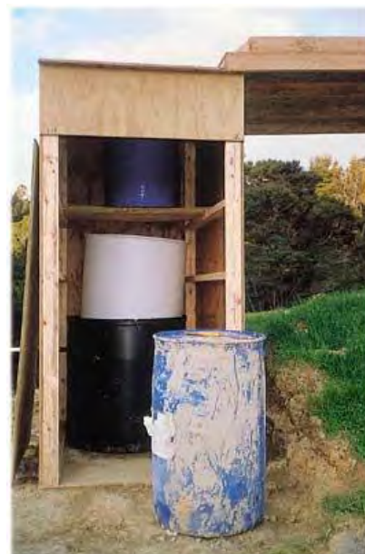
Figure 100: Rainfall activated flocculant treatment device
