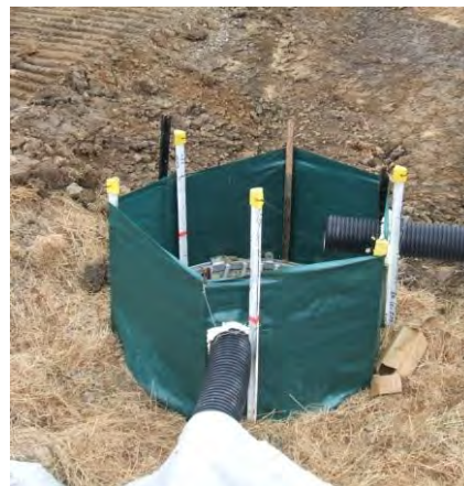
Figure 98: Good use of a silt fence installed to protect a new stormwater catchpit where impounded water will not create a flooding hazard
