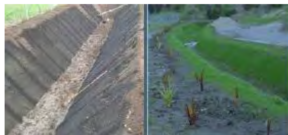
Figure 64: Bonded synthetic fibre mat used as erosion protection and medium for revegetation
