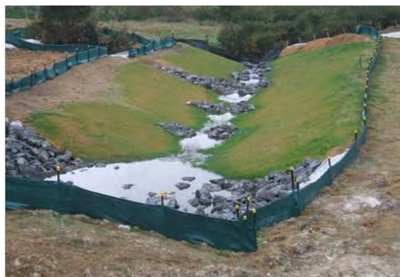
Figure 26: Check dams installed in series to act as a permanent water velocity control measure
