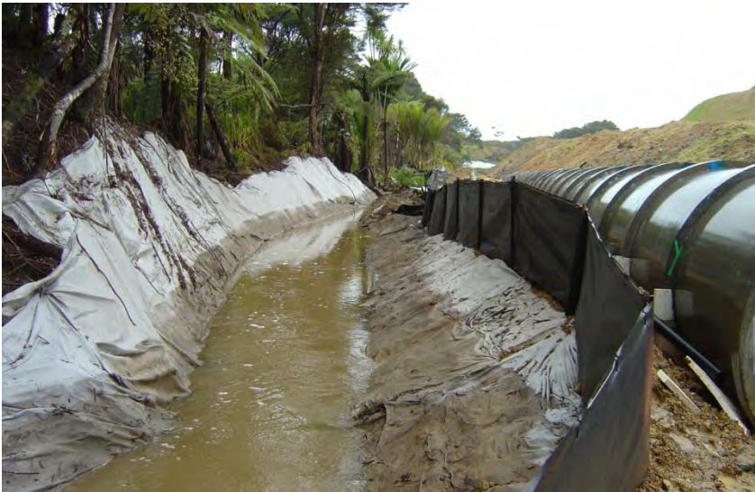
Figure 112: Temporary stream diversion to allow for the installation of a new culvert
