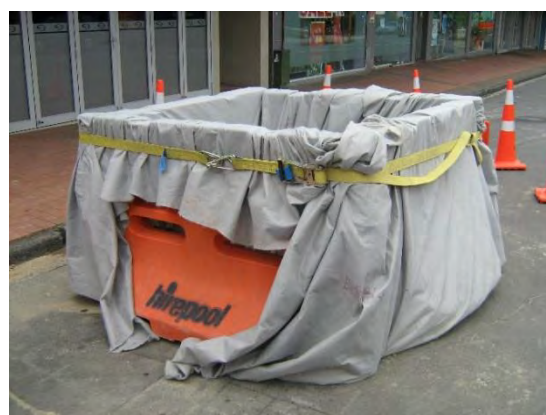
Figure 107: Example of a mobile 'turkey nest' used for dewatering
