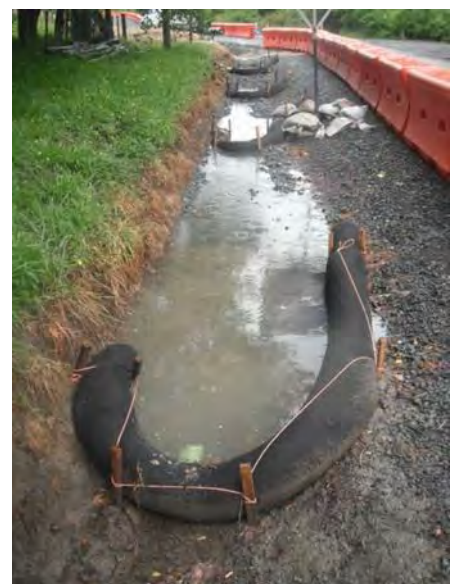
Figure 27: Silt socks can be used as a check structure on a low gradient channel
