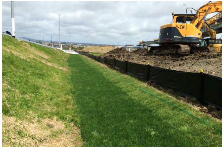
Figure 53: Turf used to provide instant stabilisation of the swale allowing for early commissioning of the device
