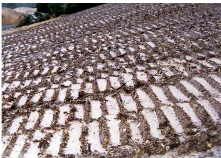
Figure 40: Surface roughening of a slope. Note the hollows acting as "micro" sediment traps
