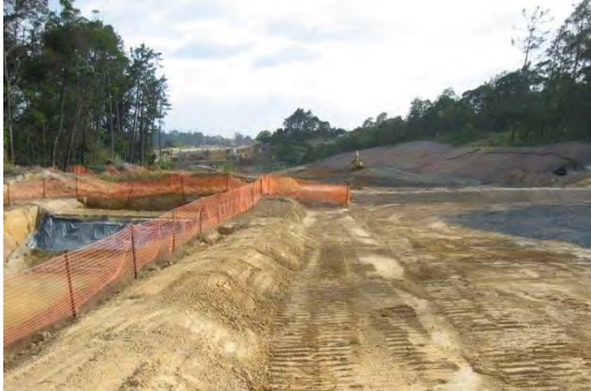
Figure 20: Dirty water diversion bund directing site water to a sediment retention pond
