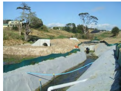
Figure 113: Stabilised clean water diversion and temporary culvert to divert streamflows while a new culvert is being constructed
