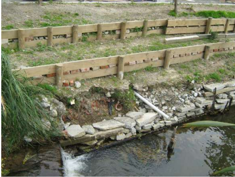
Location M. Recent bank erosion. Concrete slabs placed to attempt to mitigate further erosion.
