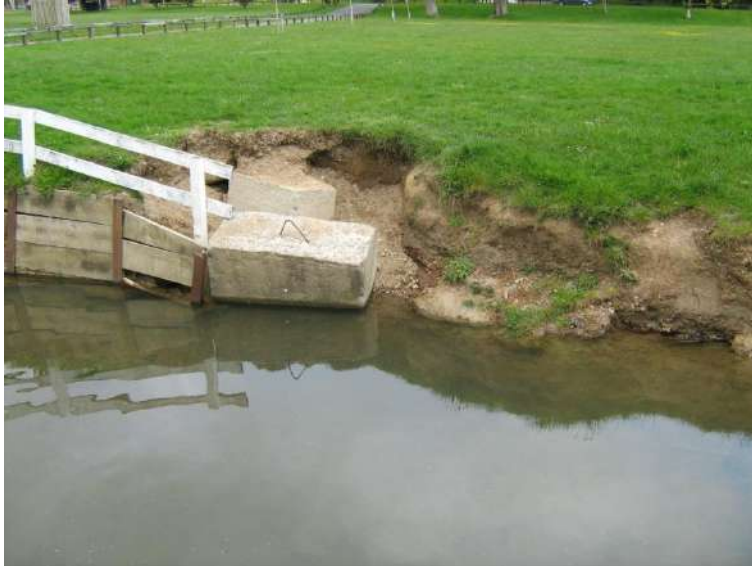
Location A. Western bank downstream of culvert. Note failure of retaining wall.
