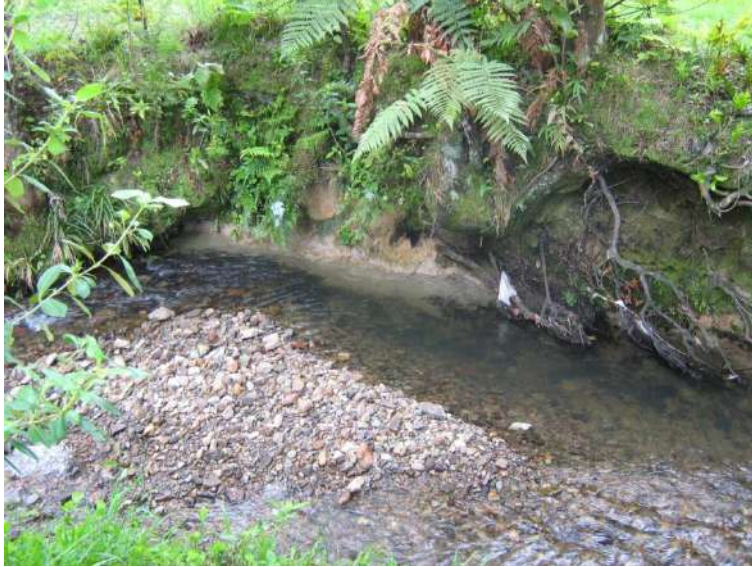
Location D. Undercutting of bank on left side of photo. Overhanging grass/topsoil on right side of photo
