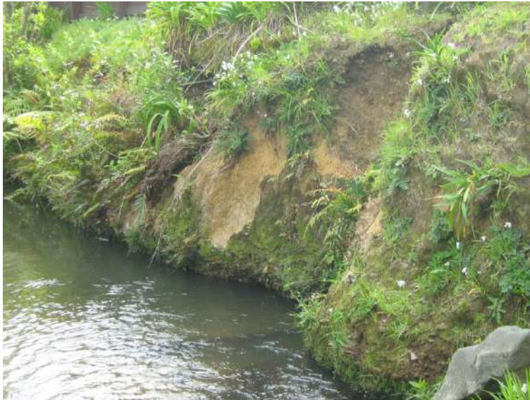
Location L. Recent bank slip.
