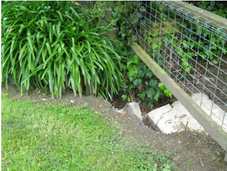
Location I. Erosion of grass above culvert on Sunbrae Drive due to overtopping.
