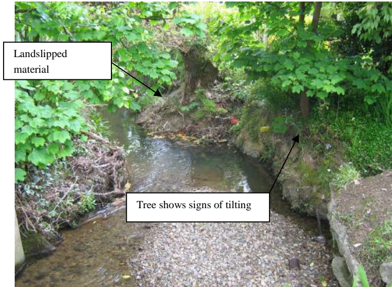
Location I. Landslip top centre of photo.
