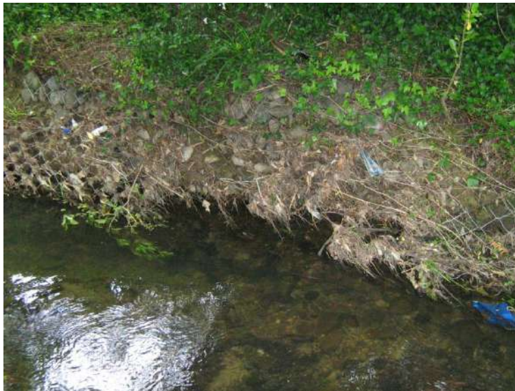
Location J. Undercutting of bank exacerbated due to failure of retention system.
