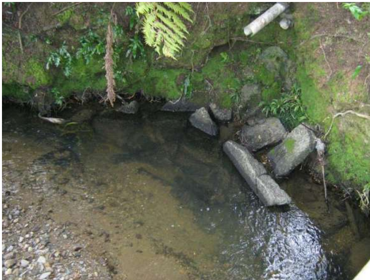
Location G. Erosion of bank due to drainage pipe. Concrete blocks placed at base of stream.
