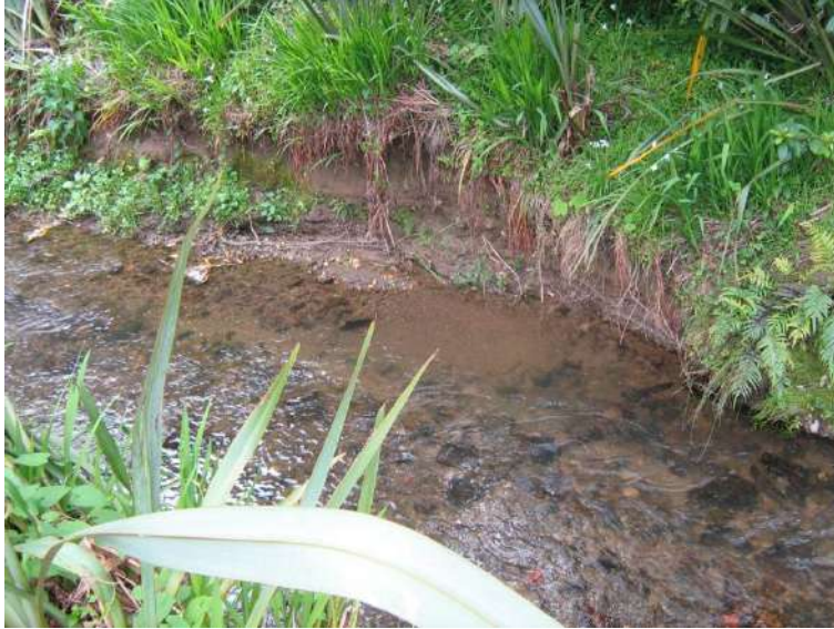
Location H. Erosion of bank at base of Pinehaven Road
