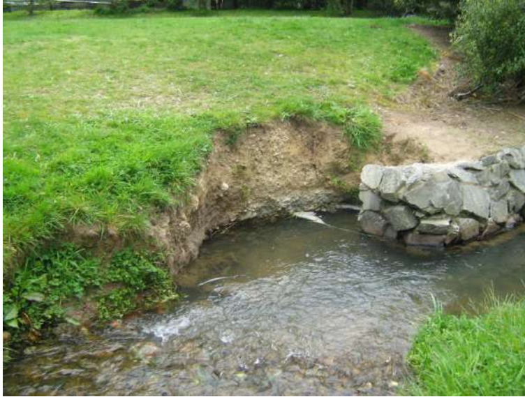
Location B. Erosion upstream of block wall
