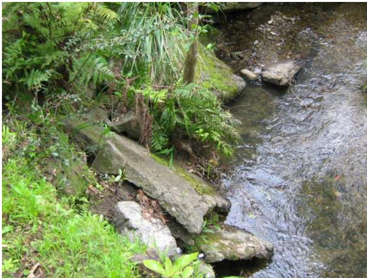
Location E. Concrete blocks at base of stream to mitigate further erosion.
