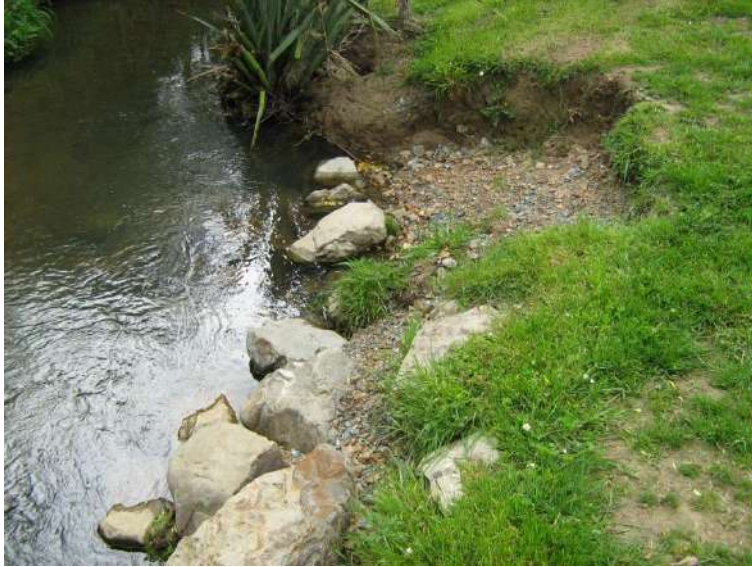
Location K. Erosion of bank mitigated by gravel fill and boulders placed at base of bank.
