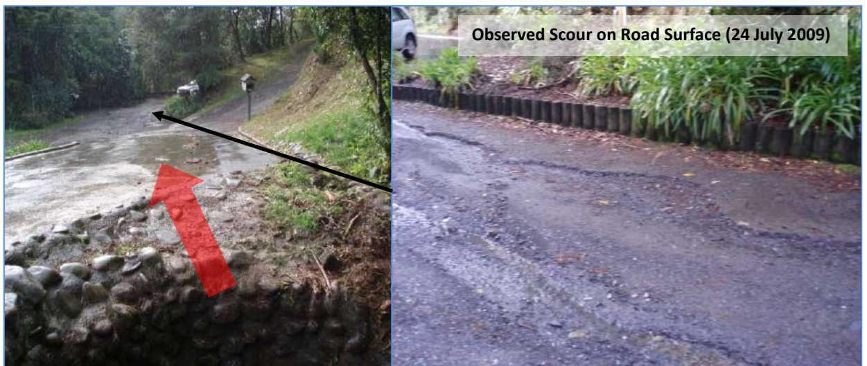
■ Figure 21 Overflow Path at the Top of Pinehaven Road
