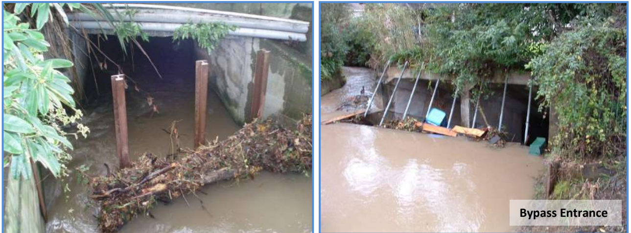
■ Figure 34 Entrances to the piped section of Pinehaven Stream and the Whitemans Road bypass as photographed following the 23 July 2009 storm
