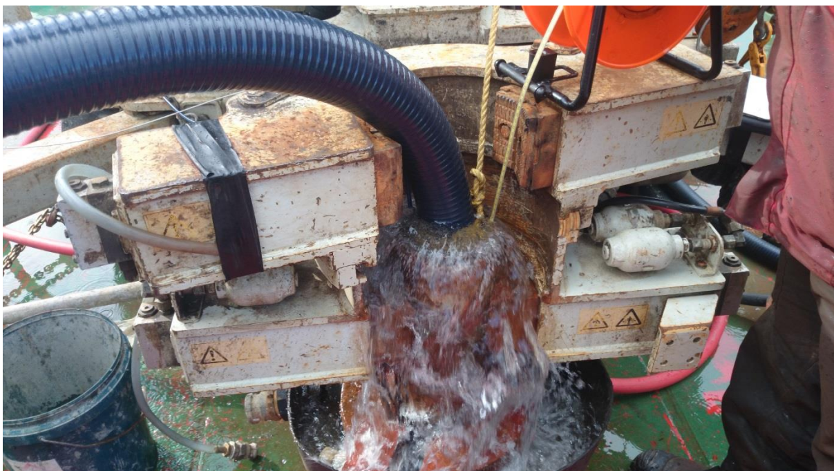
Water overflowing bore when pump turned off
