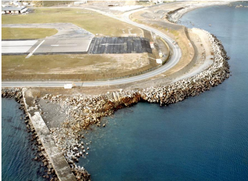
Photo 8: June 1983 seawall breach
