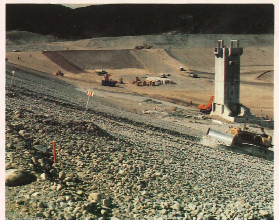
Construction of the lakes took five years from 1980. During this time work continued around the clock.
